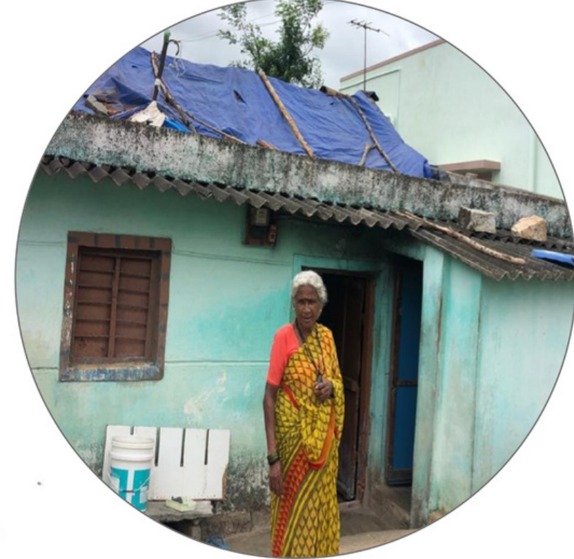
DAMAGED AC SHEET ROOF COVERED WITH TARPULIN TO PREVENT WATER LEAKAGE
