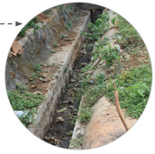
THE OPEN DRAINAGE DEPICTING THE SANITATION AND SAFETY HAZARD AMONG THE LOCALS.
