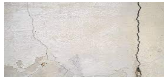
Temperature and pressure Retaining walls can develop vertical fissures in the poured concrete due to severe pressure or drastic temperature changes.
