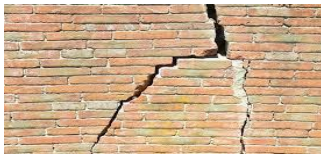
Soil pressure Some retaining walls, like brick walls, can't withstand severe soil pressure. This can lead to brick breakage or foundation failure.
