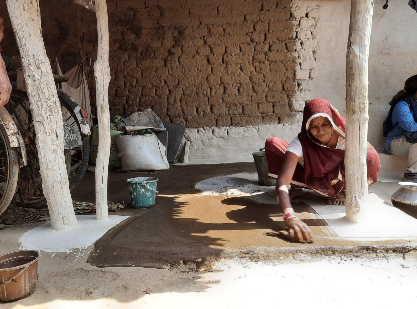
Mud-flooring artfully executed in a village in Madhya Pradesh. Barring the responsibility of incorporating foraged materials such as wood and twine, Women here not only execute finishes but also erect the super-structure through hand-made adobe blocks and roof tiles - in all of 27 days. Architecture holds potential in recognising these skills, and gender minorities as carriers of these skills through lived experience accumulated over generations.
